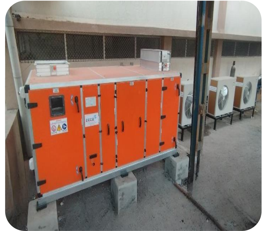
GACL – Dahej Complex HVAC solution for their Polarization 1 & 2, Store Room and Instrument Panel Room.
