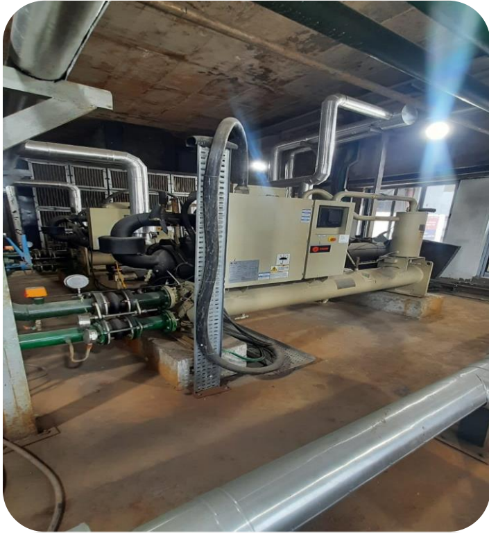
Birla Copper Dahej Turnkey solutions for their PMR Project. 72TR 2No.s Chiller with AHU of 37000 CFM, Cooling Tower of 150 TR and Pumps.
