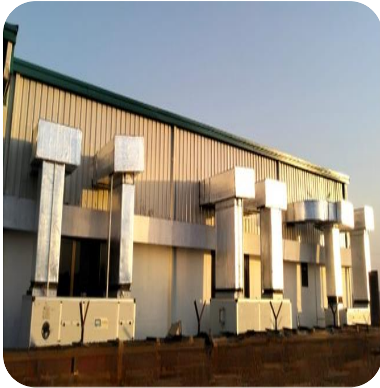
Racemosa Energy (India) Pvt. Ltd. Turnkey HVAC solution with 3 No's Air Handling Units (AHU).
