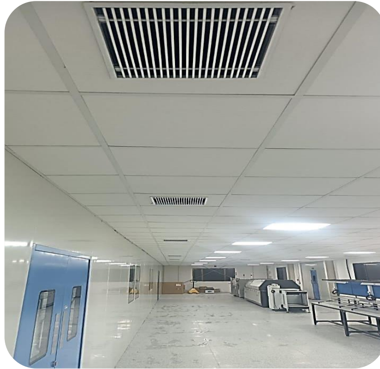
Racemosa Energy (India) Pvt. Ltd. Turnkey Clean Room solutions including design.
