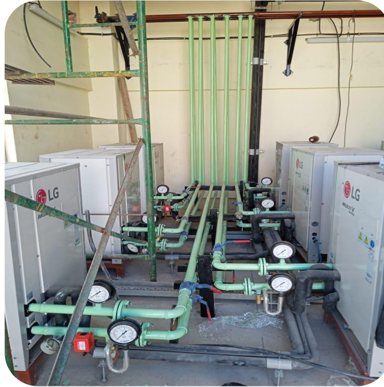
GACL – Vagra Site Dahej Turnkey solutions for their control room. 100 HP water cooled VRF System with Cassette Type Indoor Unit. Fresh Air AHU system.
